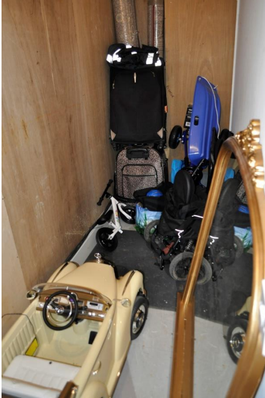
Photograph 3 – Combustible materials in electric intake room
