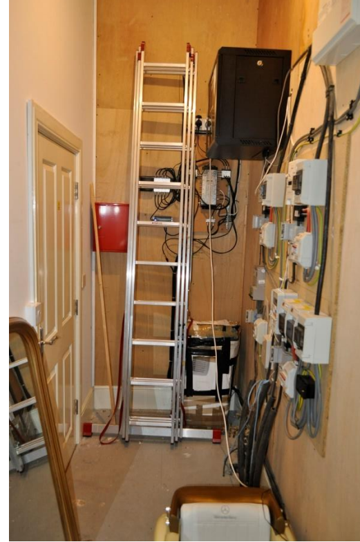
Photograph 4 – Metal ladder adjacent to electrical switch gear
